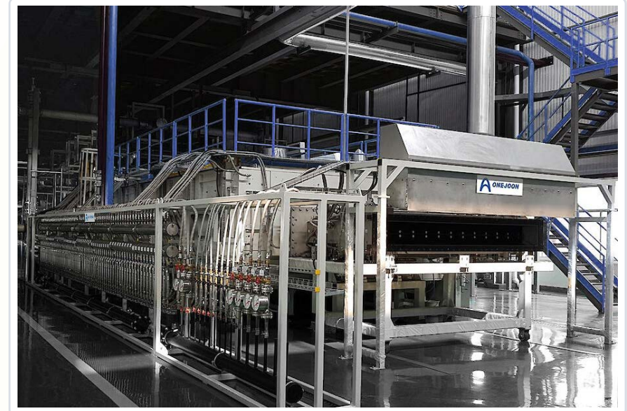
Industrial furnace example
